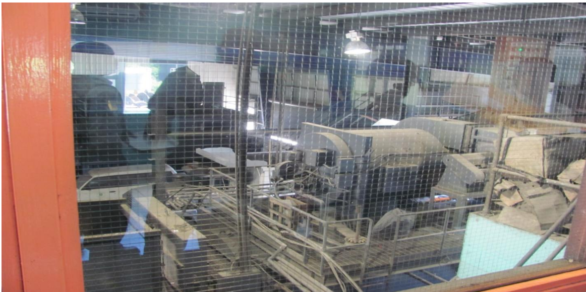
The 40 Ton incinerator.
