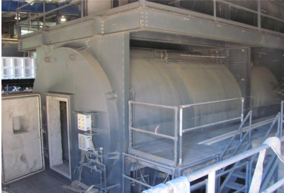
The new 100 Ton Incinerator
